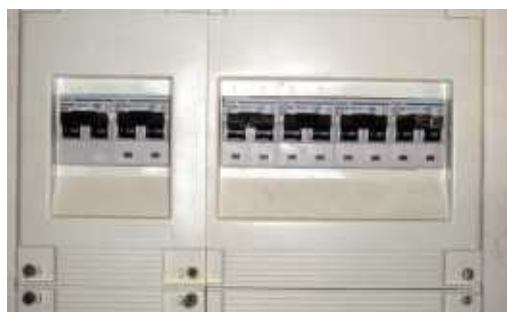
Breaker switches have their ampere rating printed on the face.
