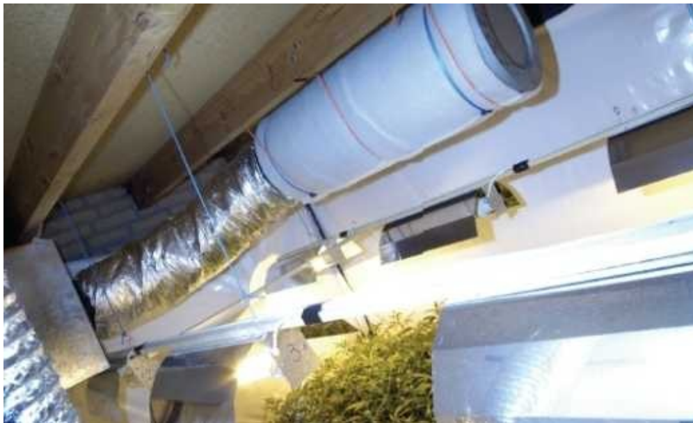
An activated charcoal filter is attached to a vent fan. The air is cleaned
