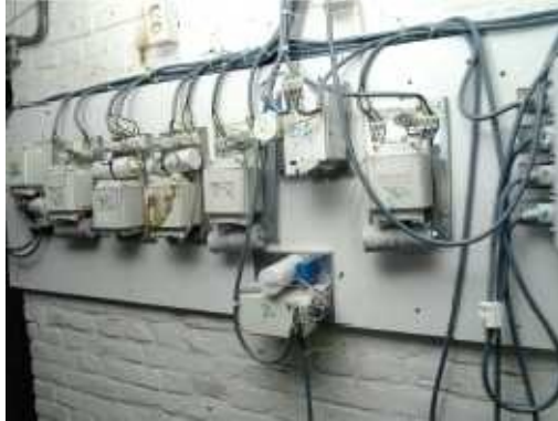
The timer on the right controls the entire lighting system in the grow room.
